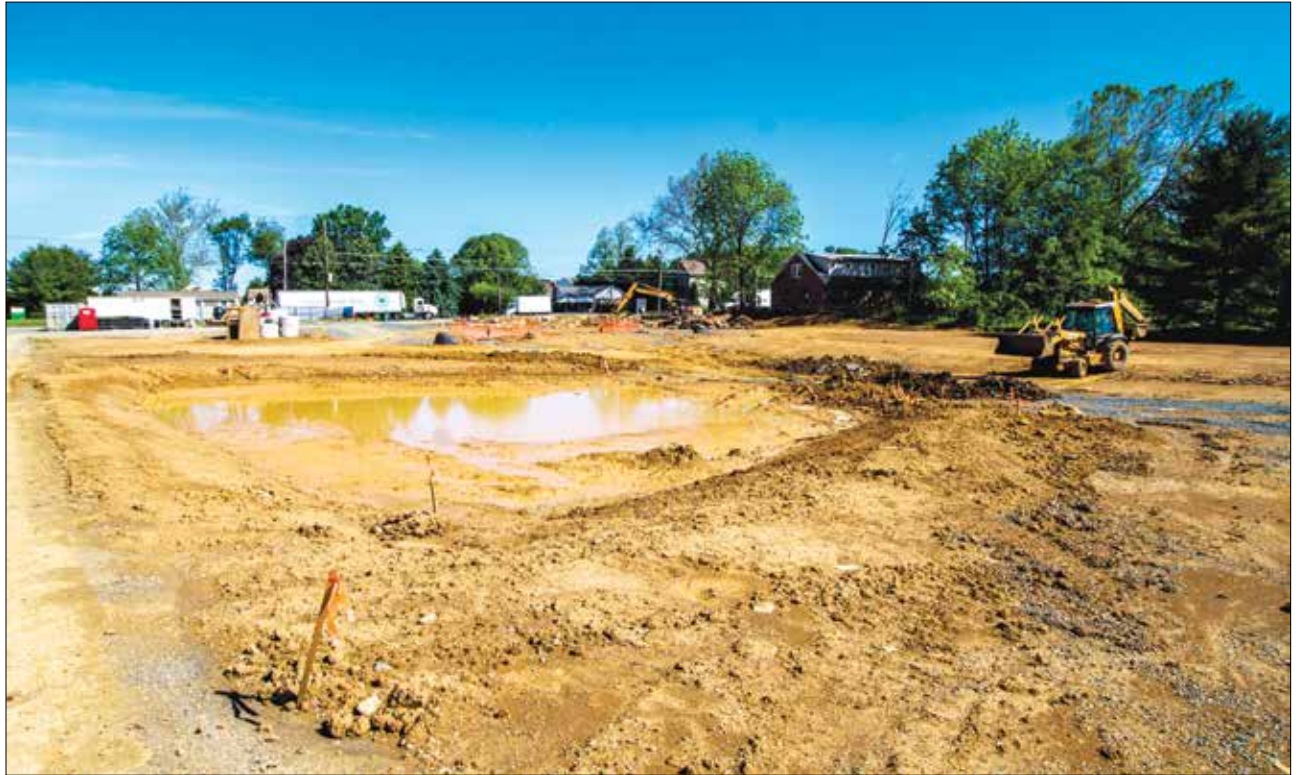
Construction is underway on The Business Park at Maiden Creek in Maiden Creek Township, Berks County. PHOTO/CHRISTOPHER HOLLAND
